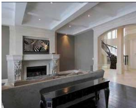
APW Custom Home Theatres of Canada performed this installation featuring Leon's HzUT-LCR ultra-thin three-channel soundbar. Courtesy Steve Pomerleau Photography.
